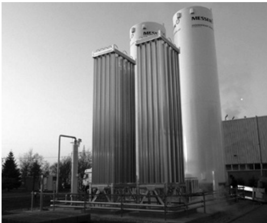
The EcoVap process harnesses the waste cold from the vaporisation of liquid gases and uses it to improve the efficiency of industrial cooling processes. Image courtesy: Messer
